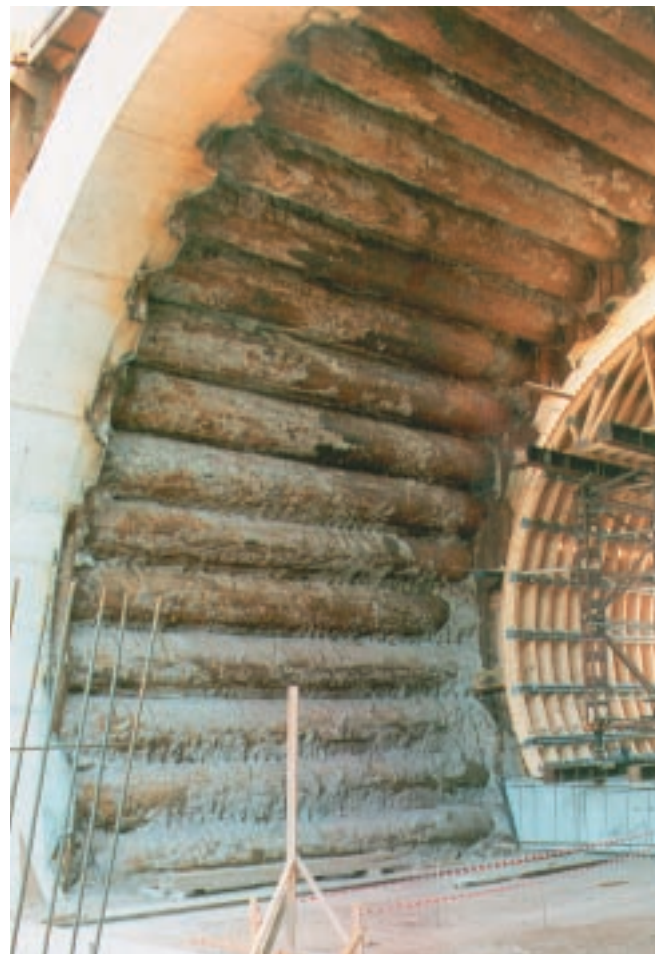
The emptied tunnel. In the background you can see the coasting carriage for producing the concrete sections.
