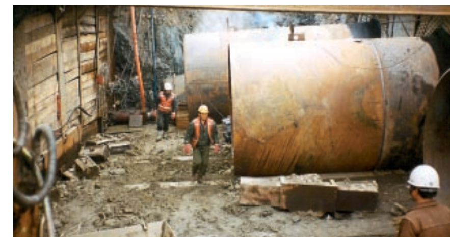
The three water pipes ND 3000 above which the "pipe roof", consisting of 39 steel pipes interconnected by special profiles, was installed.
