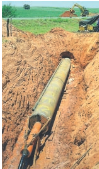
GRUNDORAM KOLOSS ramming the steel pipe ND 1000 over a length of 72 m under a highway.
