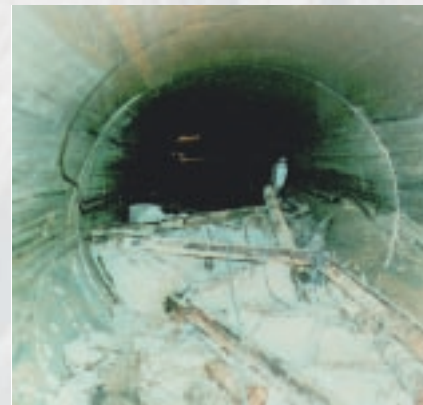
Looking through the advanced steel pipe. You can see parts of the crossing railway tracks clearly; they have been destroyed and pushed into the pipe.
