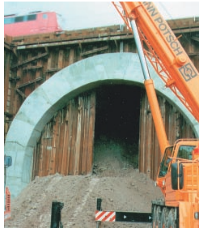
The wall is cut open in the center and excavating can begin.
