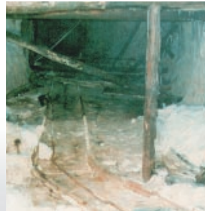
Looking into the tunnel from within the advanced pipe. No one had set a foot into the tunnel for more than 12 years.
