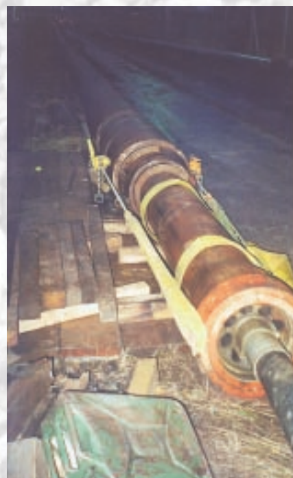
The KOLOSS pipe ramming machine at the end of the pipe string.
