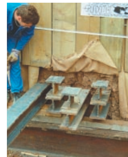
Installed IPB beams 180 mm lying on IPB beams 500 mm. The short beam part welded on is intended for beating out the beams after transplantation.
