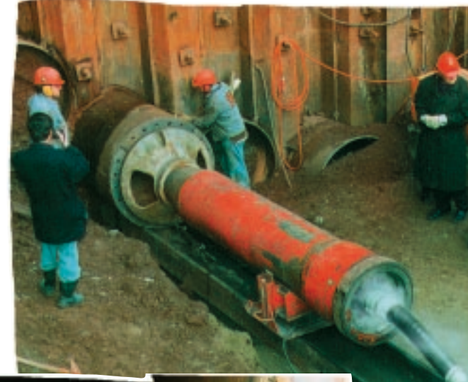
Right: The complete circle of pipes in January 1995. Below: "Topping out ceremony": TAURUS installing the last meters of pipe, December 12th 1994.
