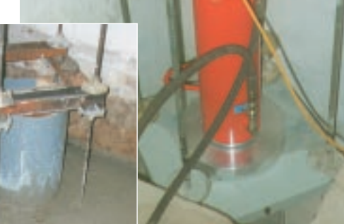
Pile foundation in practice in the cellar of a house. The facing picture displays the hydraulic press.
