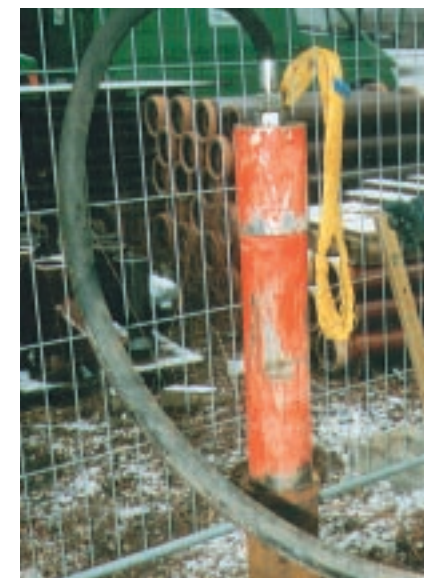
The conical steel pipe, vertically driven in by the GRUNDORAM, type MINI-OLYMP, to determine the pressure bearing capacity. The applied "wings" allow the next piece of pipe to be easily assembled and welded on.
