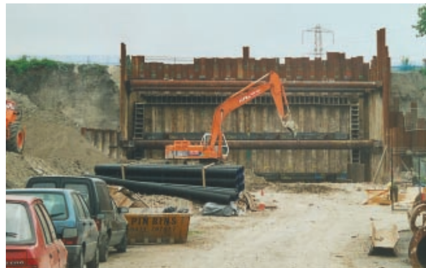
The overall jobsite view where the underpass road would eventually be excavated.
