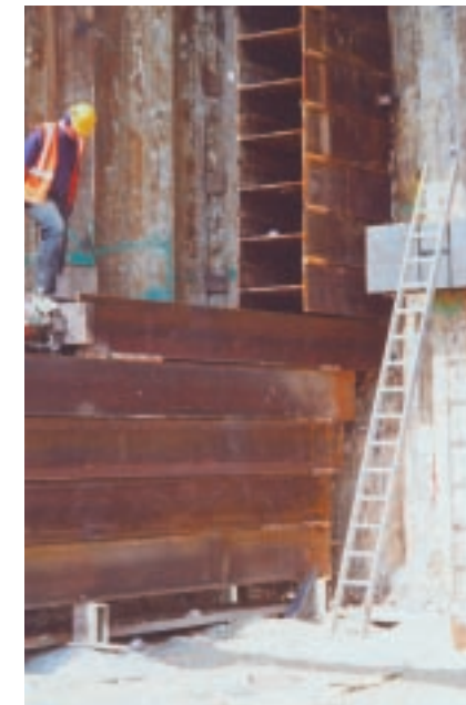
The Koloss in full operating mode where on average each beam was installed in only 45 minutes.
