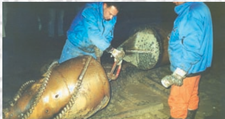
Immediately before pulling in the pipe. The pipe string is connected to the backreamer.
