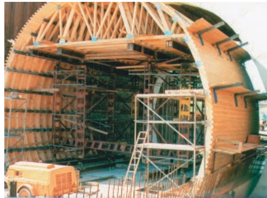
The single concrete sections (thickness 70 cm) were produced with supporting frames and a coasting carriage. Later the sections were pushed in with a hydraulic press. The carriage was loosened and driven out for the next section.
