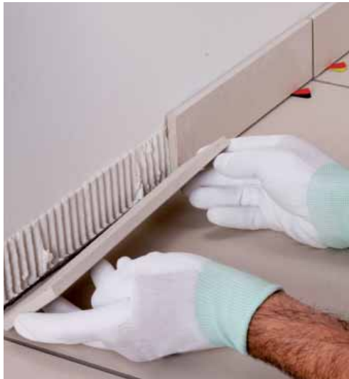
Apply the skirting around the room without letting it come into direct contact with the floor
