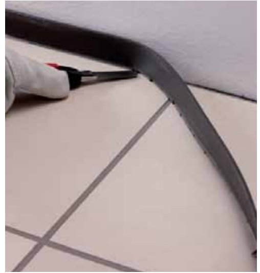
Once the grout has hardened, trim the perimeter of the Mapesonic Strip to remove the excess
