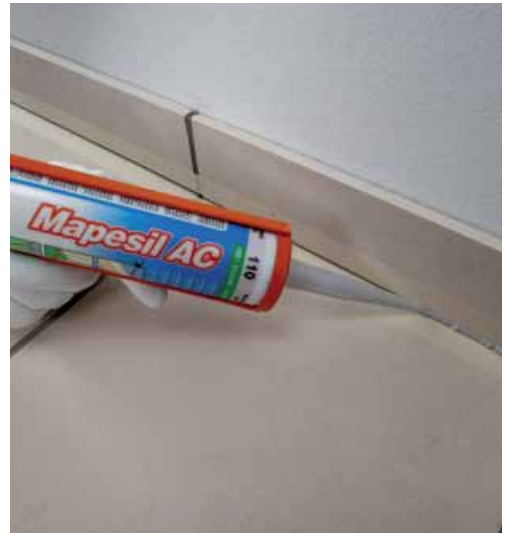
Seal the gap between the skirting board and the floor with a suitable flexible sealant from the Mapei range
