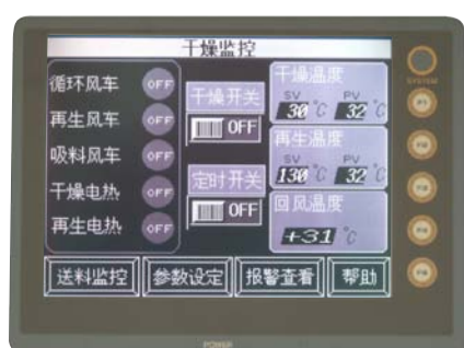
Drying process screen
